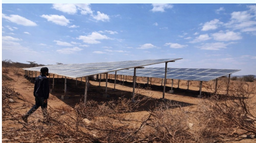
60kWp solar panels installed to power the fully solarized, climate-resilient water distribution system.
