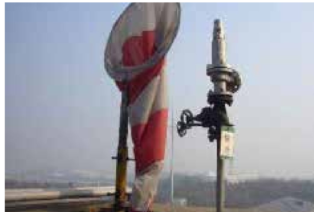
Relief valve with insufficient support and manual valve
