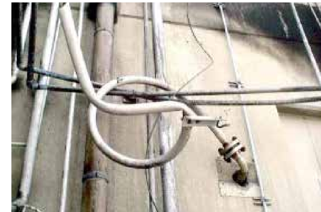
Bended relief line caused by an explosion and insufficient support
