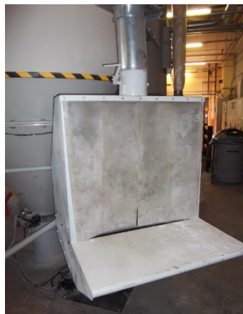
Photograph 1: Sack rip and tip station (with mechanical ventilation and shelf)
