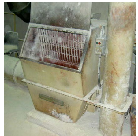
Photograph 2: Sack rip and tip station (no ventilation or shelf)
