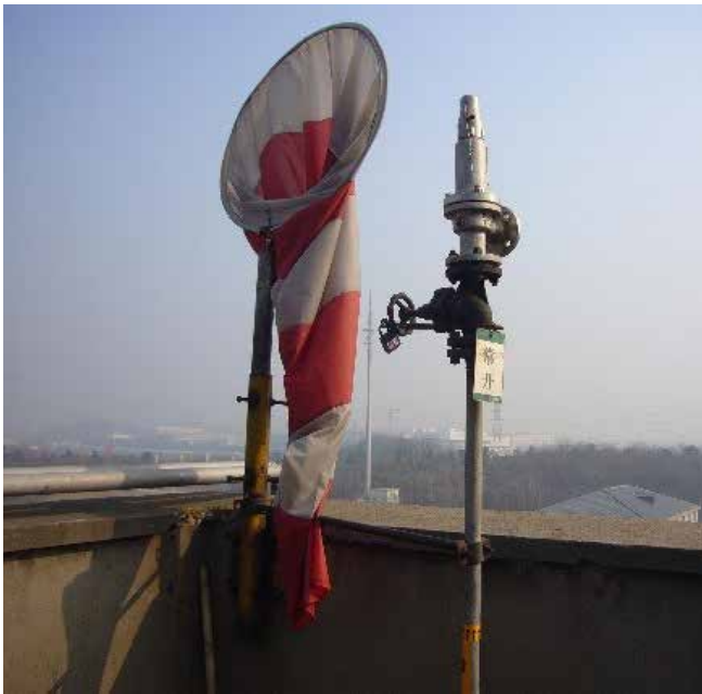
Relief valve with insufficient support and manual valve
