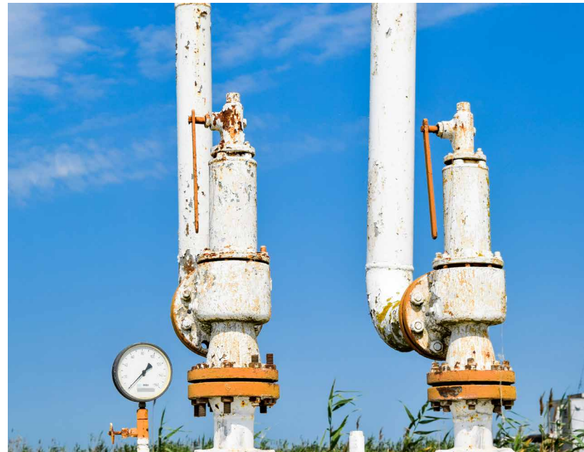
Relief valve with pressure gauge
