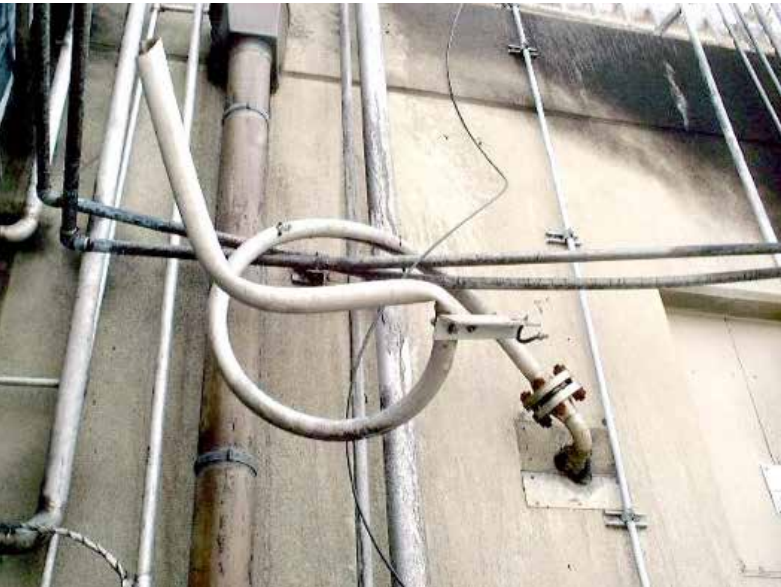
Bended relief line caused by an explosion and insufficient support
