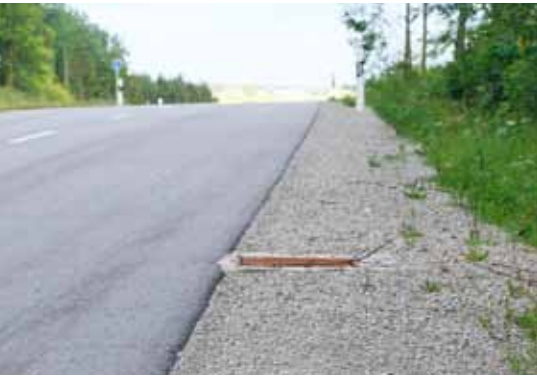
A sufficiently wide hard shoulder at the same height as the edge of the road ...
